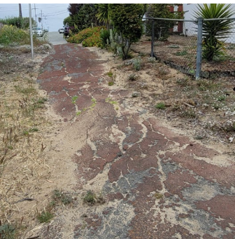
Aged Infrastructure (sitewide)
